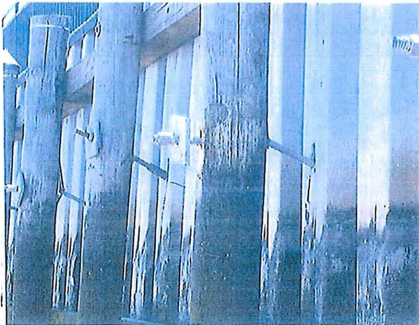
Photograph 4 - Tie rods broken; note shearing of sheet pile flange
