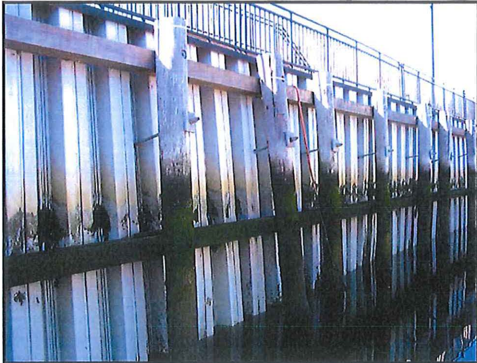
Photo No. 8 – Tie-rods placed irregularly, and at any convenient location.
