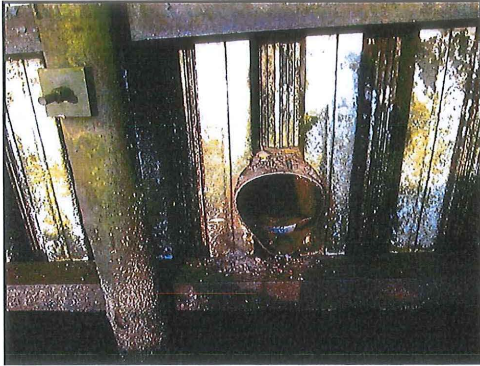
Photo No. 21 – Note loss of soil from around the 12" drain pipe.
