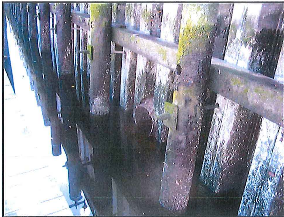
Photo No. 20 – Note loss of soil from around the 12" drain pipe.
