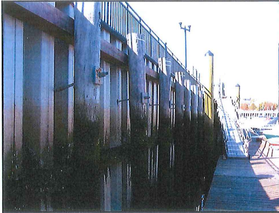
Photo No. 23 – Note slope of the tie-rods due to settlement behind the wall.
