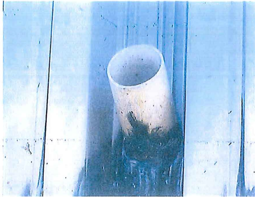
Photograph 6 - Outfall pipe sloping up
