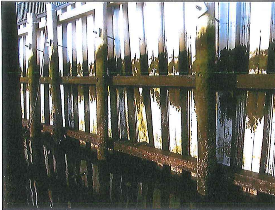
Photo No. 15 – Note skew or slope in the sheet piling. Sheet piling buckled and an additional timber block was placed.
