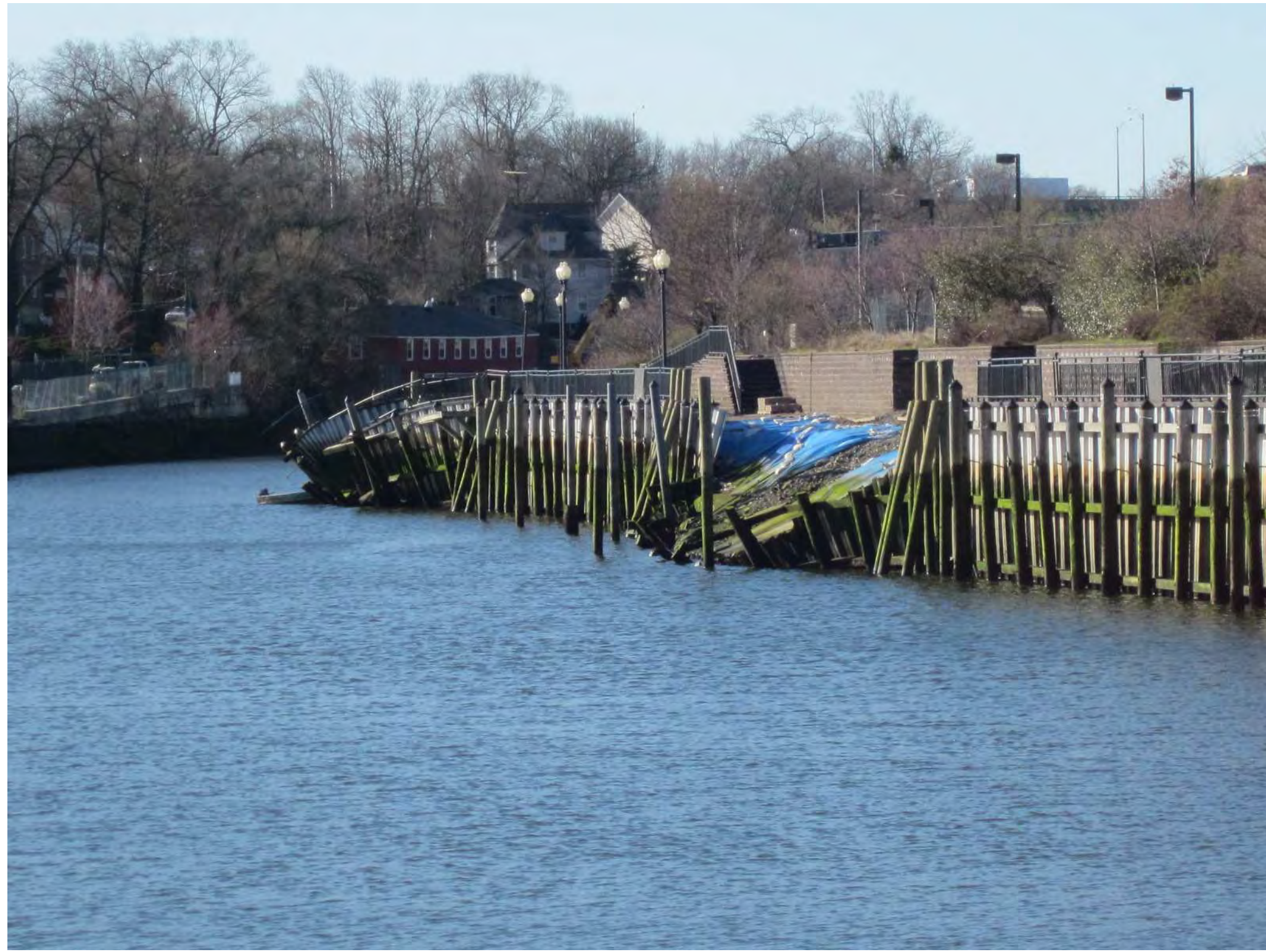
General View Collapsed Bulkhead- Looking South
