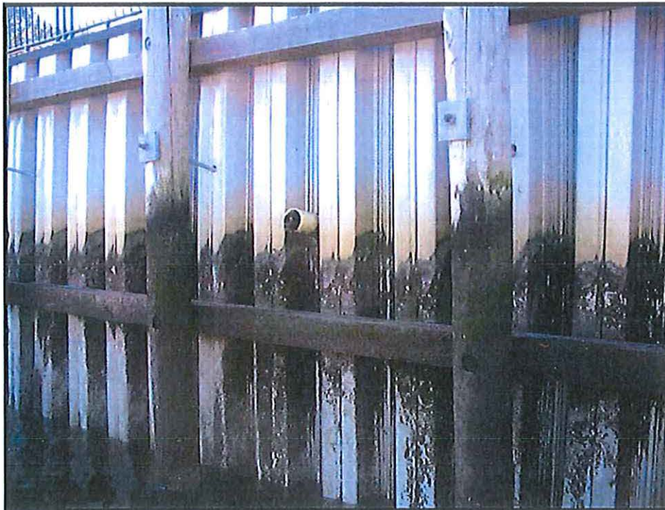
Photo No. 2 – Note the excessive downward slope in the tie-rods and weep holes due to settlement behind the wall.
