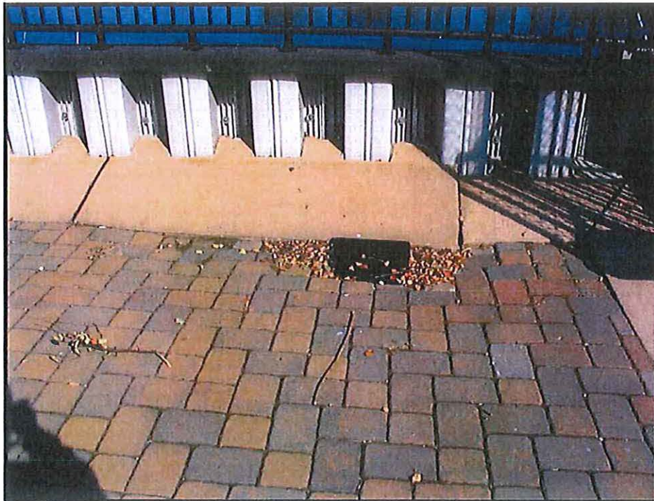
Photo No. 24 – Settlement at a storm drain at the top of the bulkhead.
