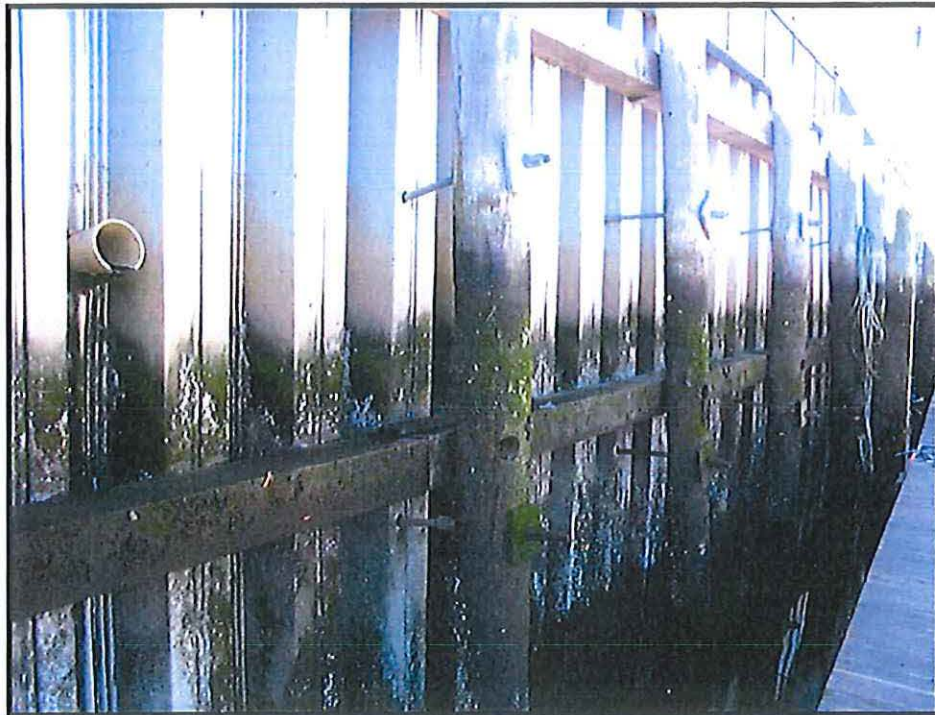
Photo No. 18 – Note the steep slope in tie-rods and weep holes due to settlement behind the wall.
