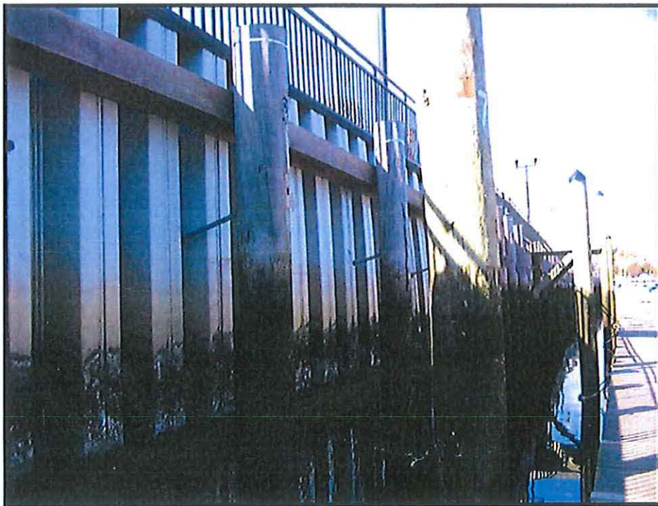
Photo No. 4 – The replacement sheet pile bulkhead. Very poor construction techniques were utilized.
