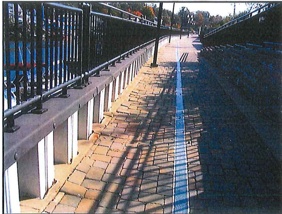
Photo No. 26 – Settlement along the storm drain at the top of the bulkhead.
