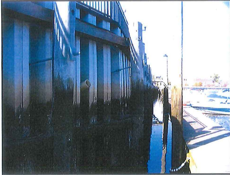
Photo No. 3 – The replacement sheet pile bulkhead. Note the steep slope in the weep hole due to settlement behind the wall.
